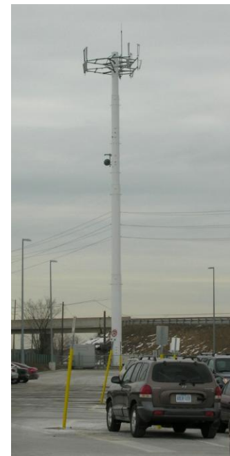
Cell Tower – Mount Pleasant GO Station
