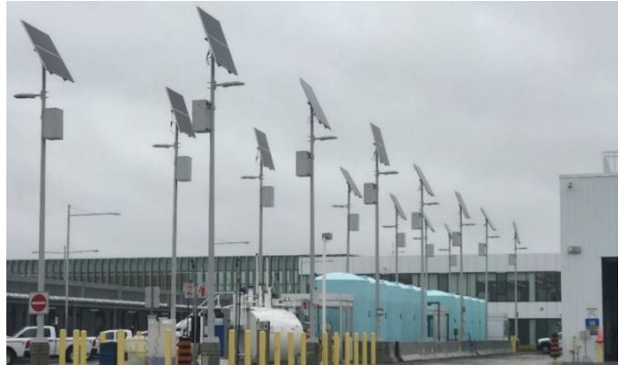
Figure 11 Solar-Powered Lighting System installed at Williams Parkway Operations Centre
