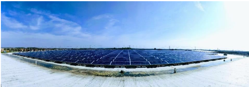
Figure 9 Panoramic shot of solar PV system at Cassie Campbell Community
