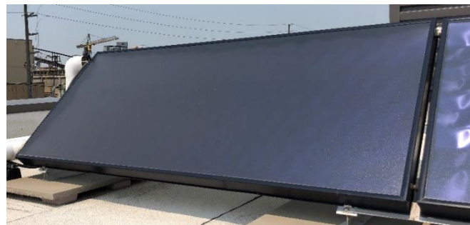
Figure 10 One of four solar collectors that are a part of the solar thermal system installed at Brampton Apparatus and Maintenance Facility
