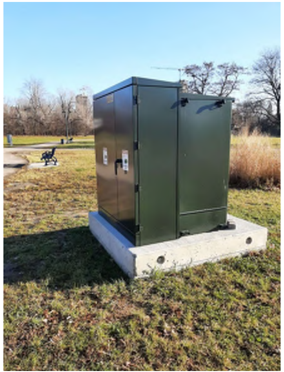
Photograph 8: Transformer located at northwest entrance of the Site.
