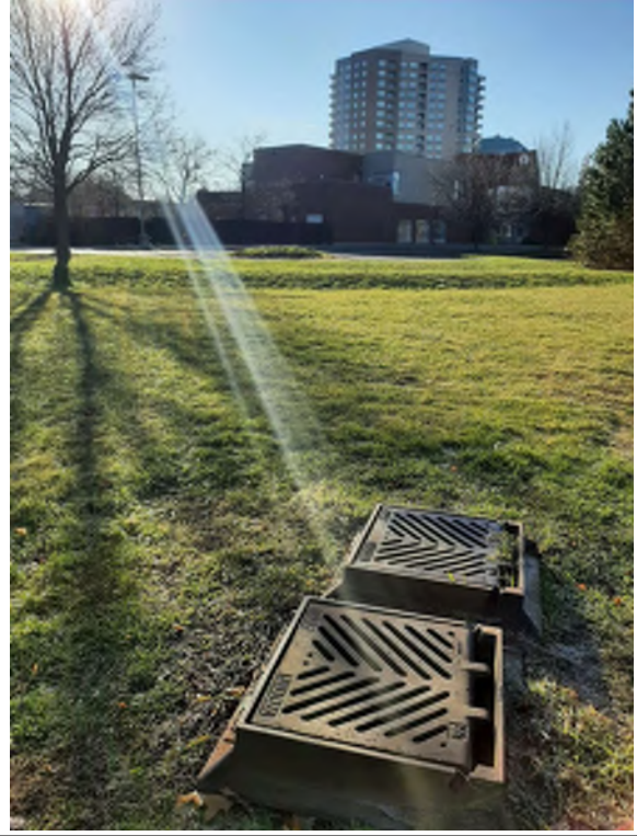
Photograph 6: On-site catch basins located in the central portion of the Site, west of the roundabout.
