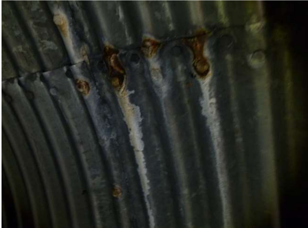
PHOTOGRAPH 9 CULVERT BARREL - RUSTED JOINTS
