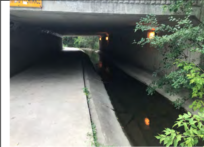
Photo 19: View of concrete lined Tributary of Spring Creek under the Williams Parkway bridge, facing south.
